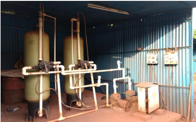
STP for treatment of Domestic Waste Water
